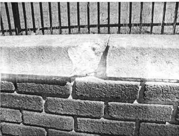
Damaged Retaining Wall Coping
