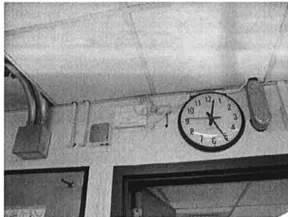
Typical Electrical Conduits
