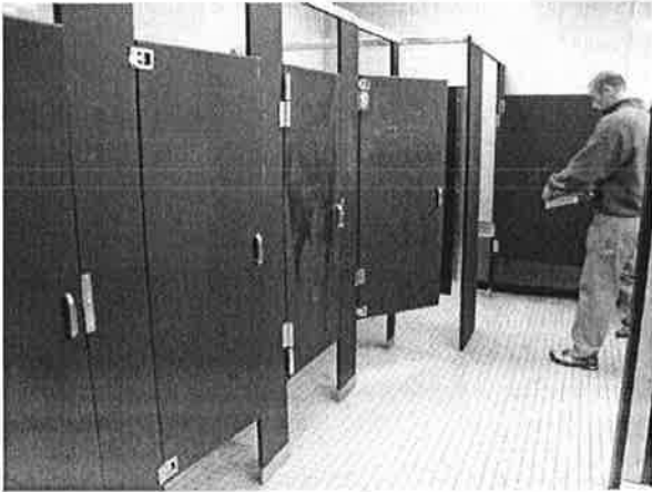
Typical Group Toilet room Stall Dividers
