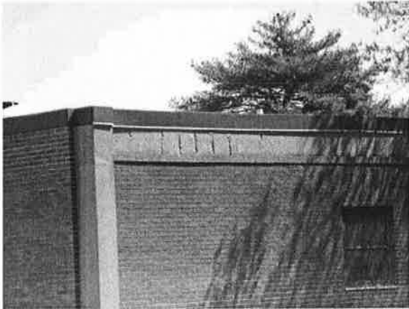
Exposed Rebar on Pre-cast Concrete
