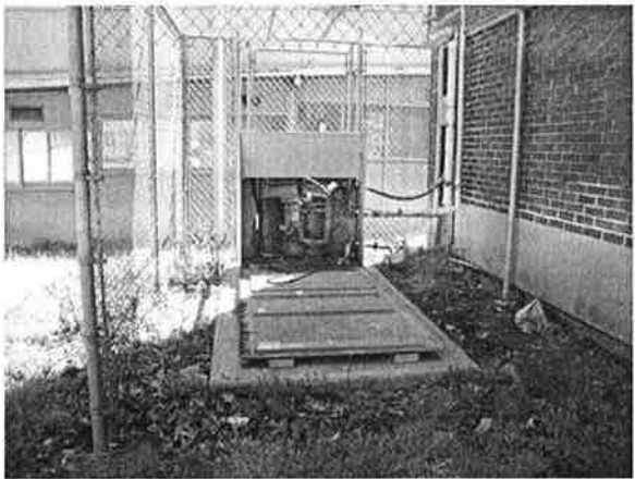
Vandalized Condenser outside Gymnasium
