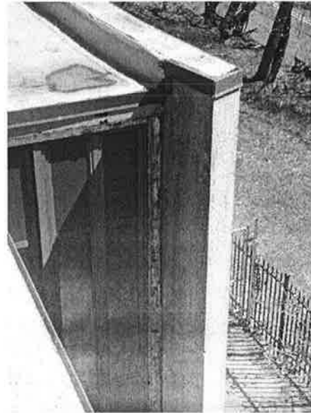
Rusted Window Lintel - Annex Stair Tower
