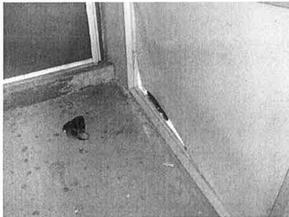
Aluminum Wall Separation in 1970 Bridge
