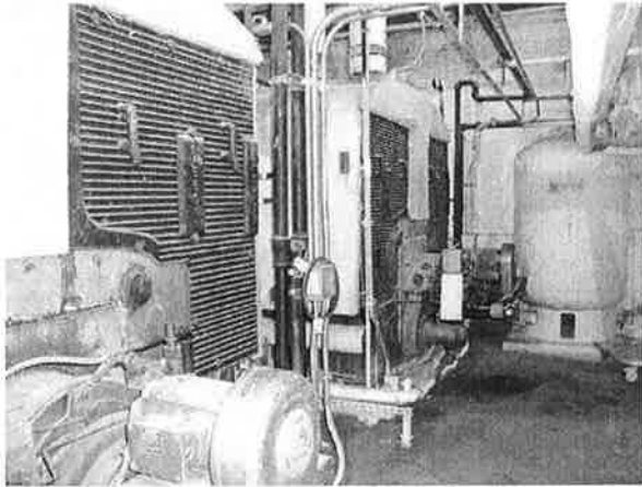
Boiler Room in 1916 Building
