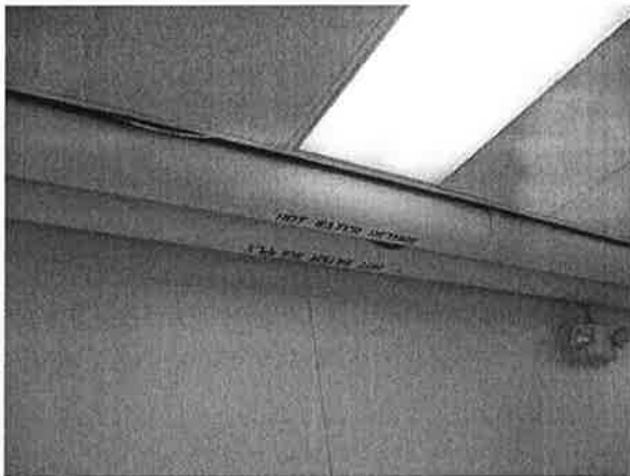
Hot Water Supply Piping in Hallways
