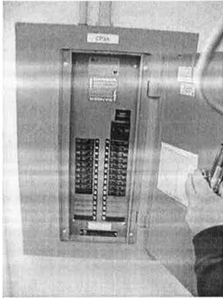
Typical Interior of Electrical Panel
