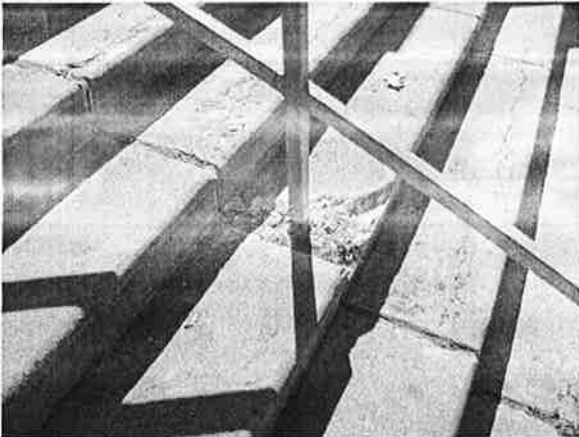
Site Handrail Needing Inspection
