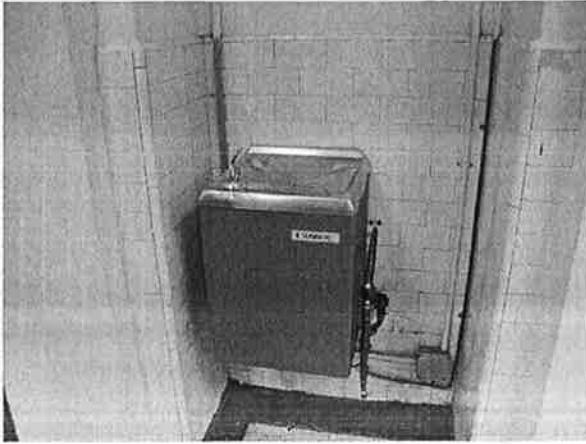
Typical Aluminum Water Fountain
