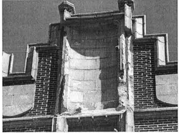
Typical Terra Cotta Deterioration
