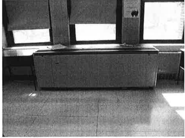
Typical Classroom Unit Ventilator
