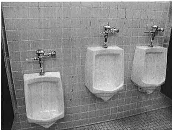
Typical Wall-Mounted Urinals
