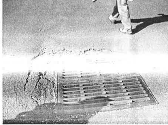
Storm Drain with Poor Paving
